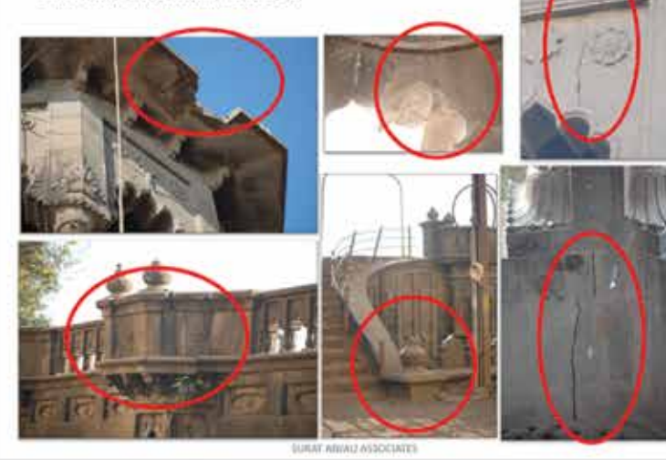
DEFECT MAPPING RANKALA TOWER
